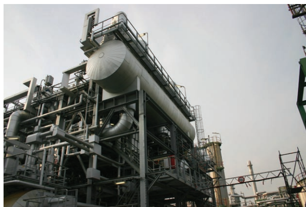
Figure 3. The new sulfur plant in Gelsenleirchen-Horst refinery with two Claus reactors and an LT-SCOT reactor in one shell.
