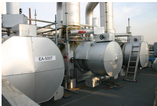
Figure 4. From left to right: Claus reheater, Claus reheater and LT-SCOT reheater.
