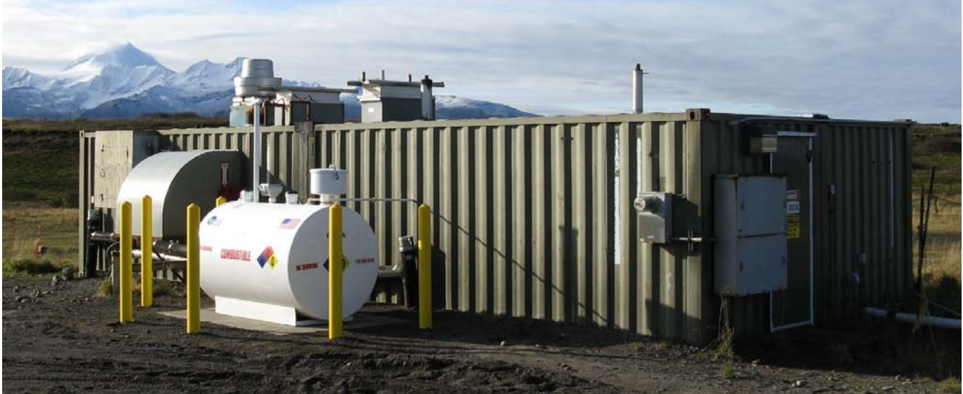
U.S. Army Engineering District, Alaska (USAED) Cold Bay Remediation Project Cold Bay, Alaska
