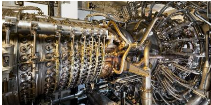
University of Texas Energy Efficiency and Microgrid Austin, Texas, U.S.A.
