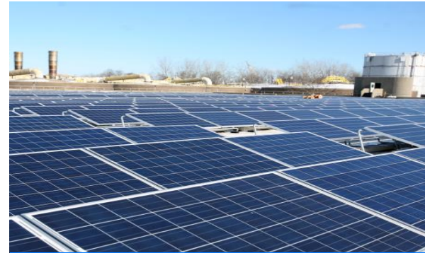
Solar Panels at Port Richmond WRRF
